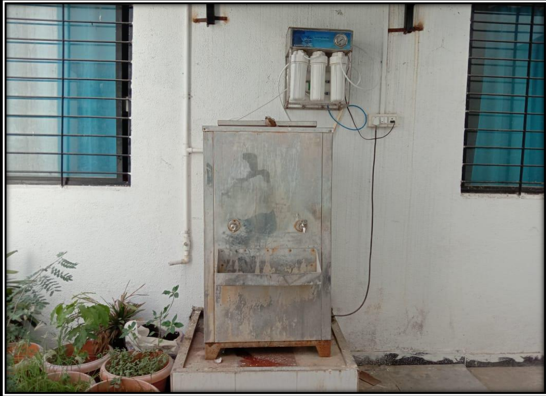
Potable Drinking Water Facility
